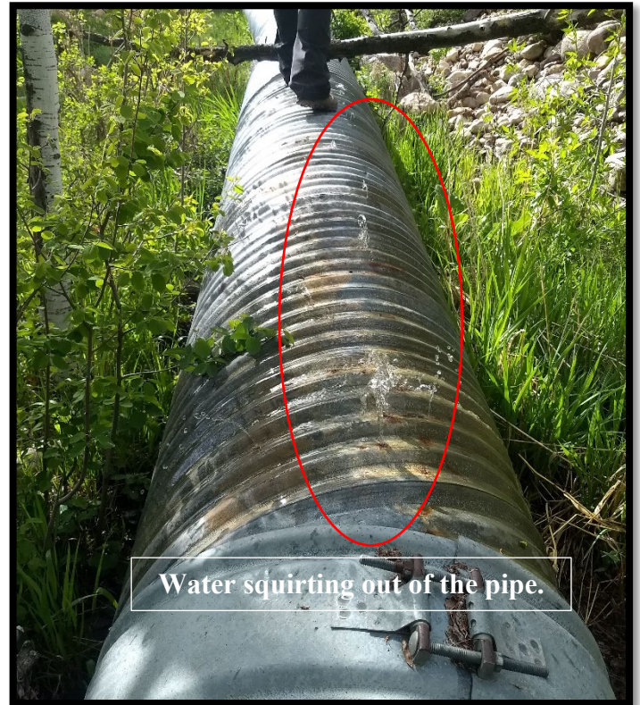
Photo 4 Water losses out of the CMP
