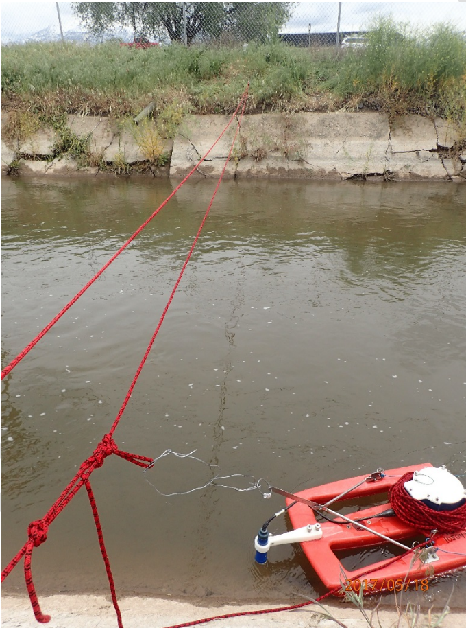
Figure 8 – Mid-stream measurement location data collection setup. Note highly fractured concrete liner. ADCP is mounted in boom position.
