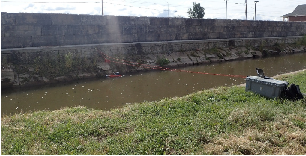
Figure 7 - Upstream measurement location. Note vegetation growing in cracks of fractured concrete liner. ADCP is in boom position.
