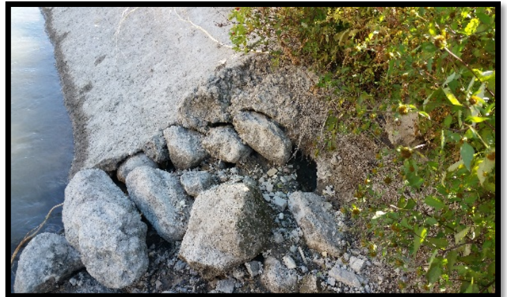
Photo 3 Broken concrete liner on the West Main Canal
