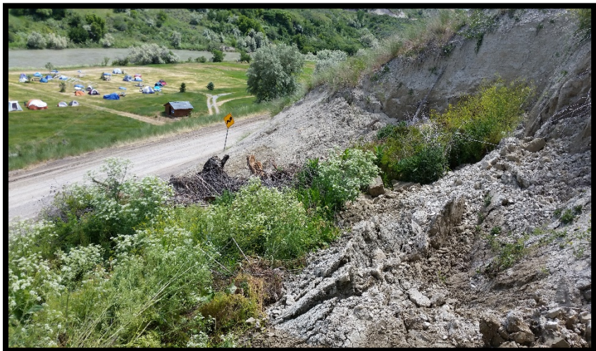
Photo 1 Canal Hillside Sluffing off/Boy Scout Camp
