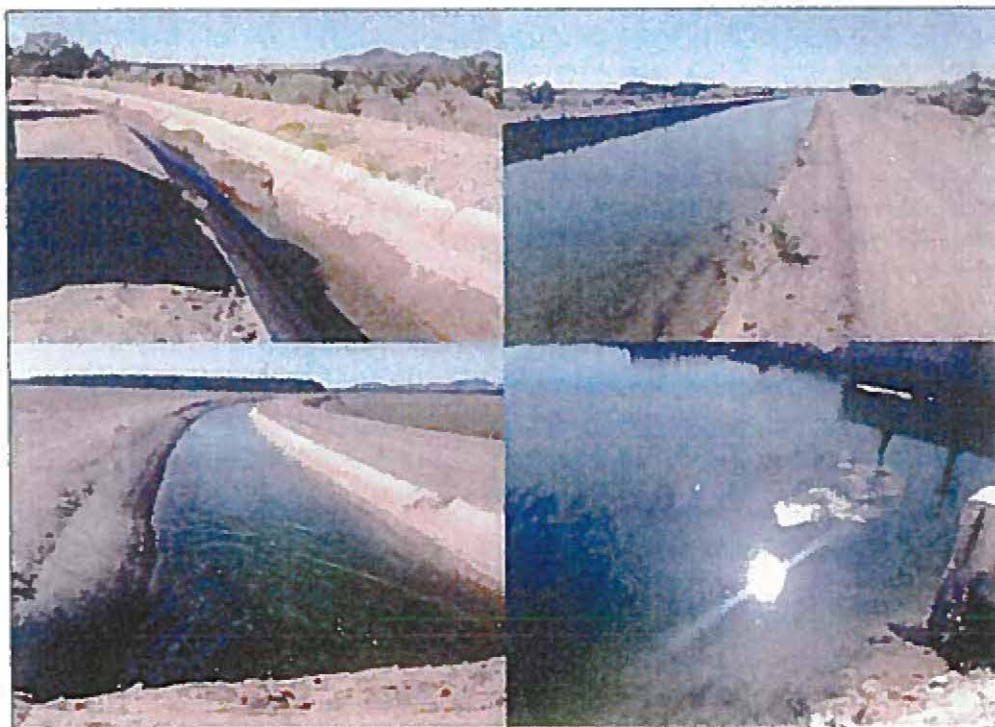
Figure 65.—Main Canal photographs highlighting sedimentation and vegetation in both unlined and lined portions of the canal.
