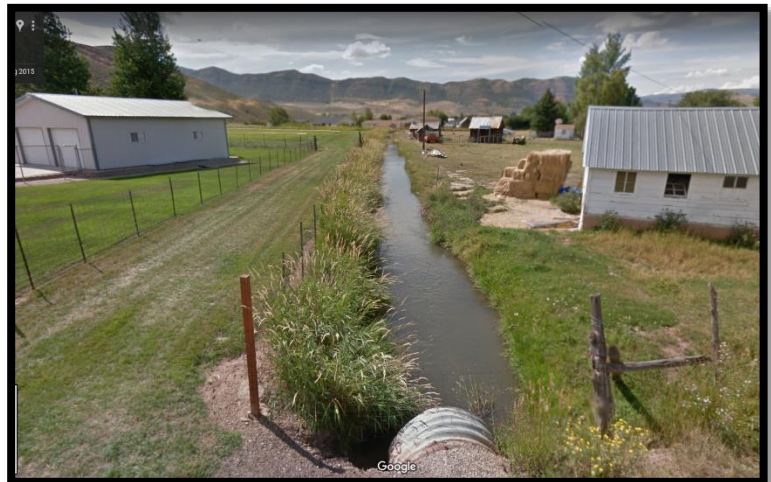
Photo 1 Main Canal that leaks and floods that will be lined
