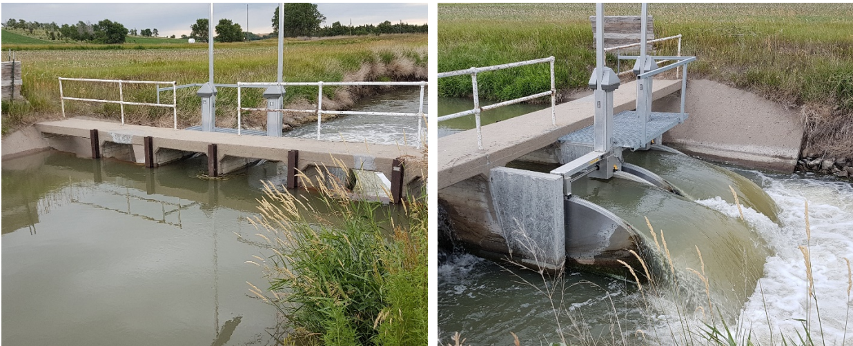
Figure 6 - FlumeGates installed into Frenchman Cambridge Irrigation District's Check Structures on the Cambridge Canal
