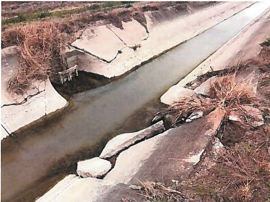
Picture 3 Failure at a service lateral west side slope (right side). The gray to white band in background at approximately 12 inches below the grass line indicates the canal's operational water surface elevation.
