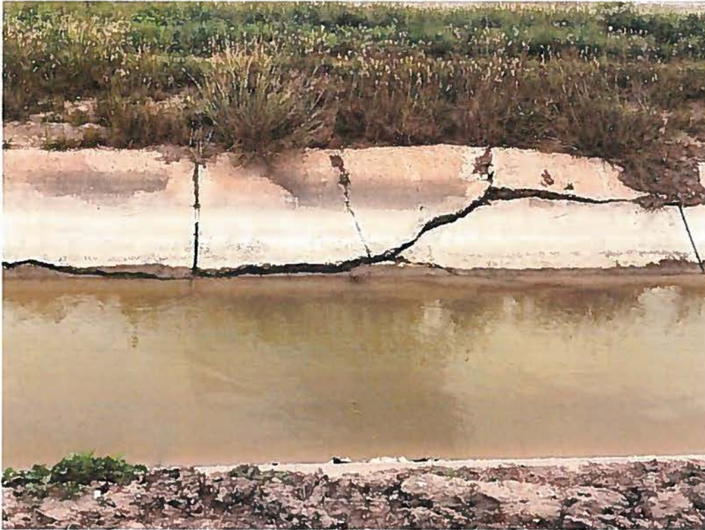
Picture 2 Visible buckling and structural movement.
