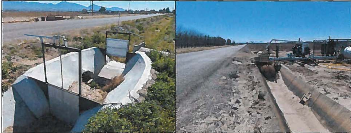
Figure 12 – Upgraded Release Gates and Concrete Lining Affected by Sediment
