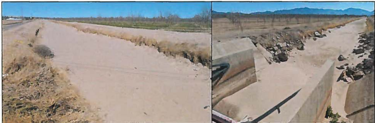
Figure 14 – Sediment Buildup at La Union East Canal after 2018 Irrigation Season
