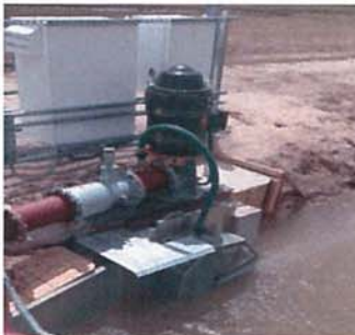
Figure 1: Existing Personal Irrigation Pumping Station
