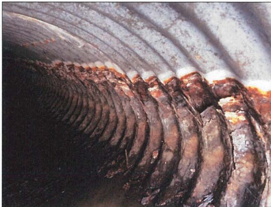
Photograph E: Rusted corrugated pipe
