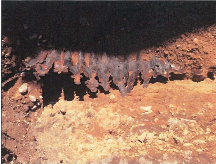
Photograph F: Rusted out bottom of corrugated pipe
