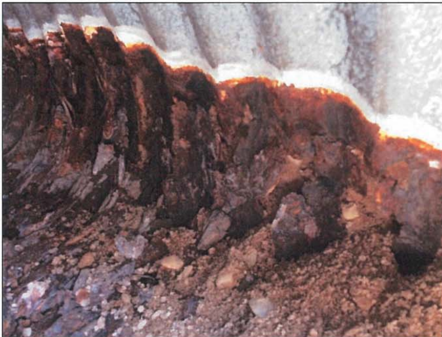
Photograph G: Rusted out bottom of corrugated pipe
