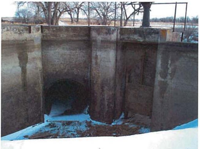
12/18/2013 IM000463.JPG Looking East (Downstream) Towards Siphon Inlet, Wasteway Gate, and Overflow Weir (on right)
