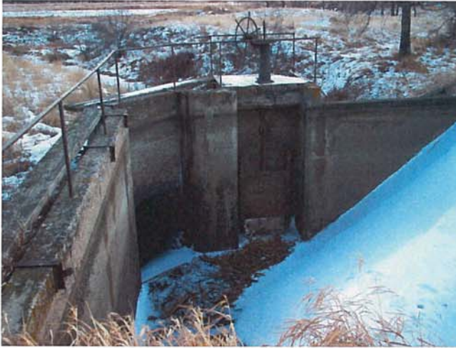
12/18/2013 IM000464.JPG Looking East (Downstream) Towards Siphon Inlet, Wasteway Gate, and Overflow Weir (on right)
