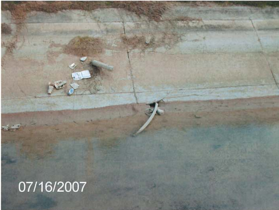
Picture 1. Visible horizontal cracks and an abandoned utility conduit.
