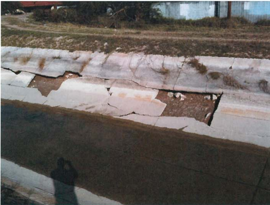
Picture 2 Visible failure of unreinforced concrete liner.
