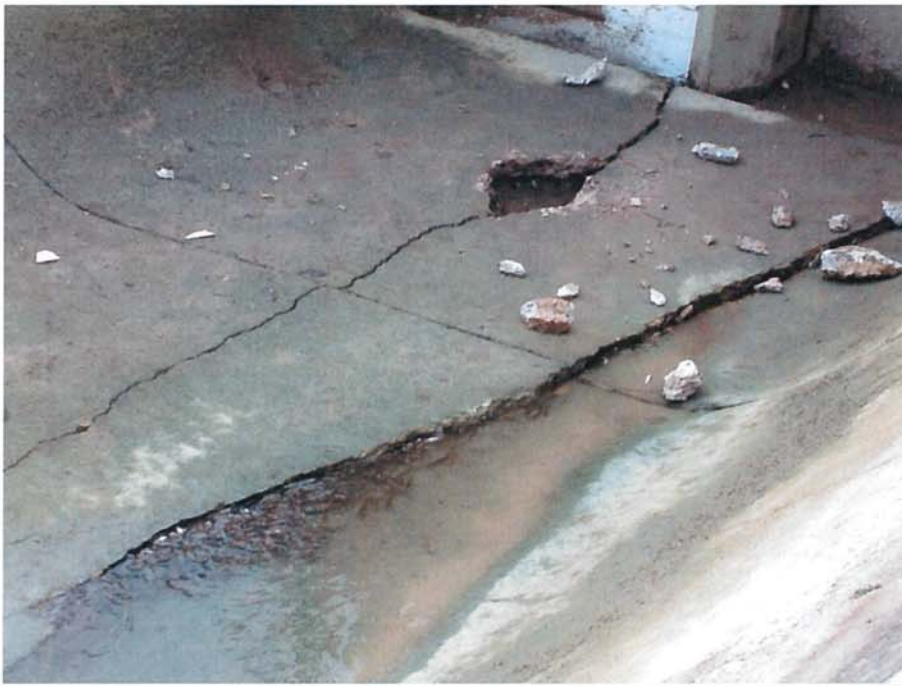
Picture 4 Broken section of liner.
