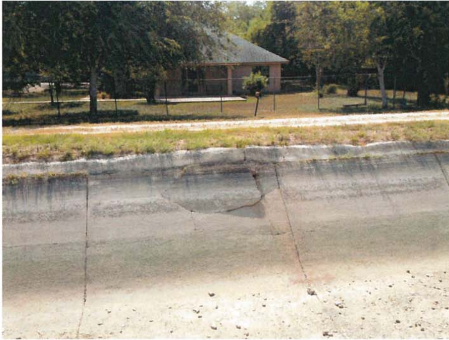
Picture 3 Longitudinal crack and a buckled section of unreinforced concrete liner.
