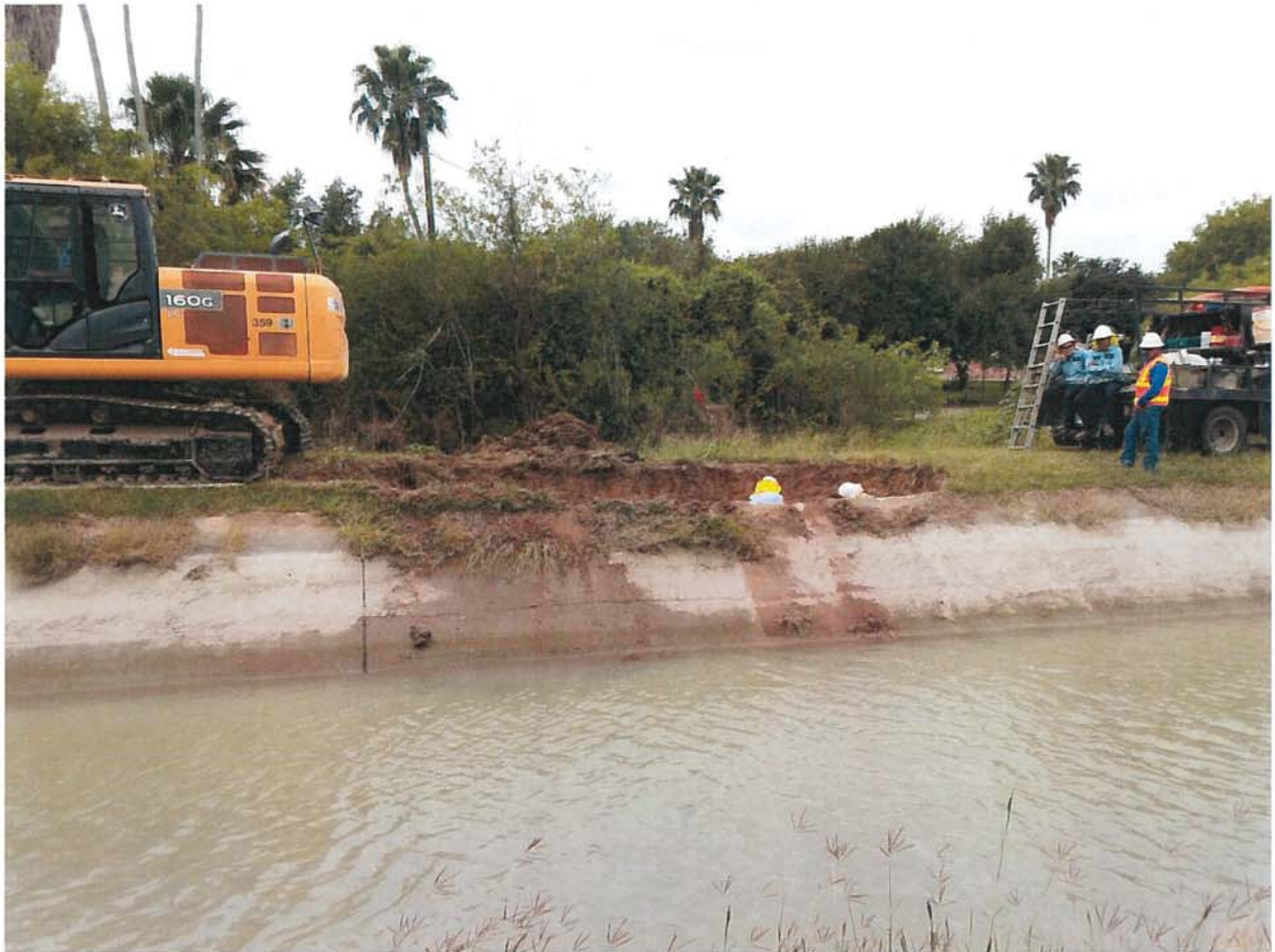
Picture 5. April 9 th , 2018 Lateral E Canal at approximately 1,200 linear feet southeast of Cage Blvd. (U.S. 281) in Pharr, Texas. Seen in the background, the District's repair crew working on a canal leak. The gray to white band in the concrete liner at approximately 12 inches below the grass line indicates the canal's operational water surface elevation.
