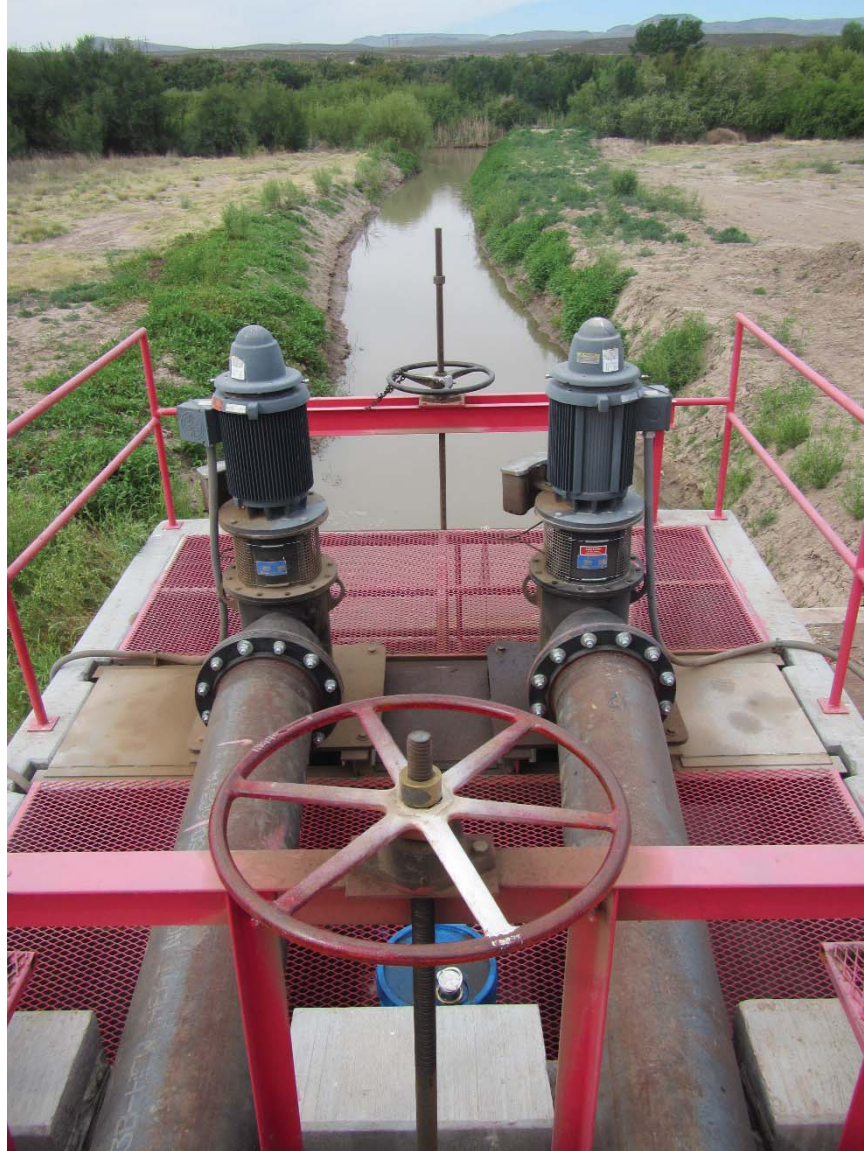
Figure 3. Pumps installed at the Rincon Wasteway 18
