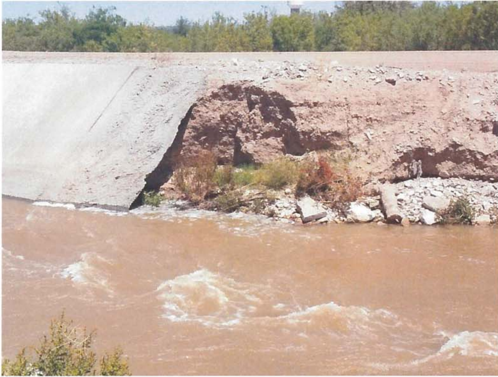
FIGURE 8 Damages to Concrete Joints at the Riverside Canal
