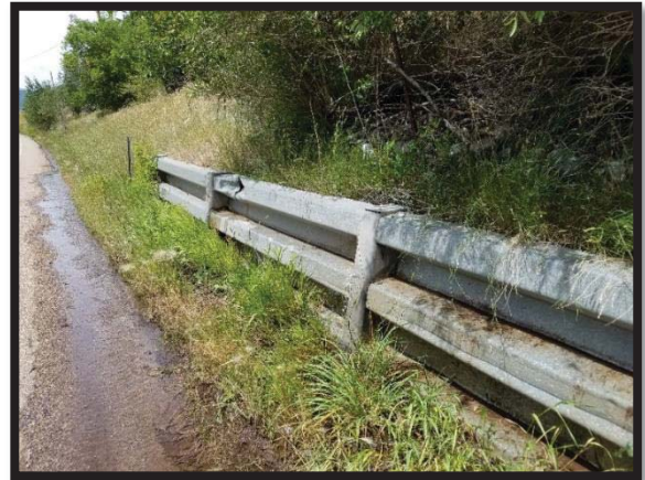
Photo 2 Water seeping into the Highway and Crossing Private Property
