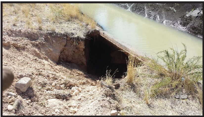
Photo 6 Canal Liner Void
