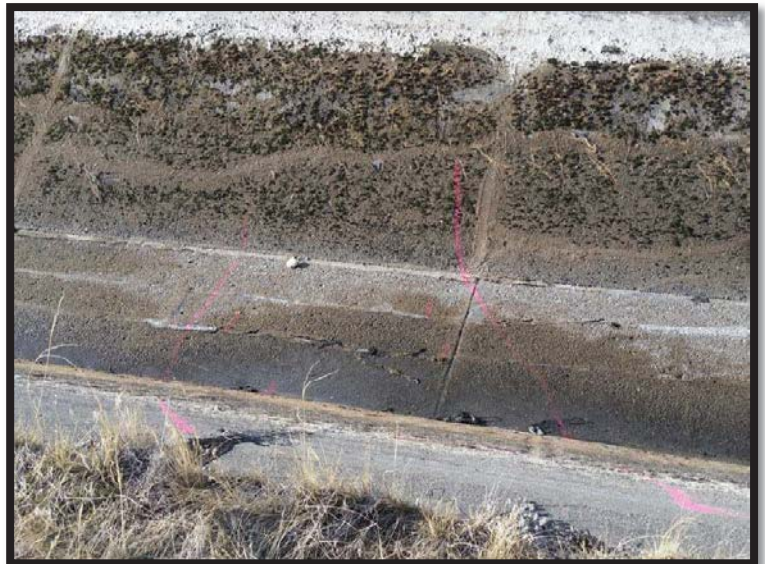
Photo 7 Cracked and broken liner
