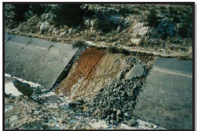
Photo 1 Breach of the Side of the canal of the Rattlesnake Liner
