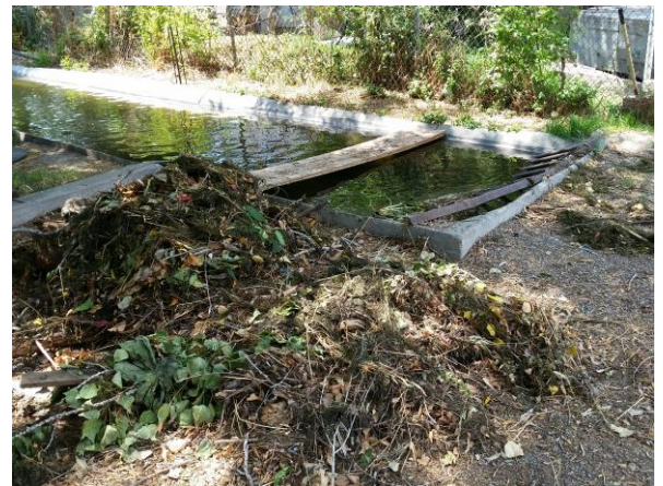
Debris must be removed manually because of the limited space available to access the canal.
