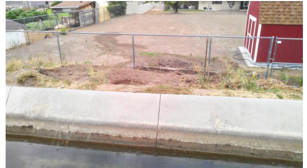
Cracking in the concrete liner causes water to seep into adjacent yards and properties.
