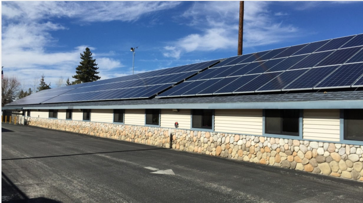
Figure 3 BBLDWP Office Solar Panels
