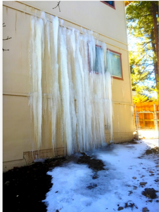
Figure 4 Home damage due to frozen and bursting pipes
