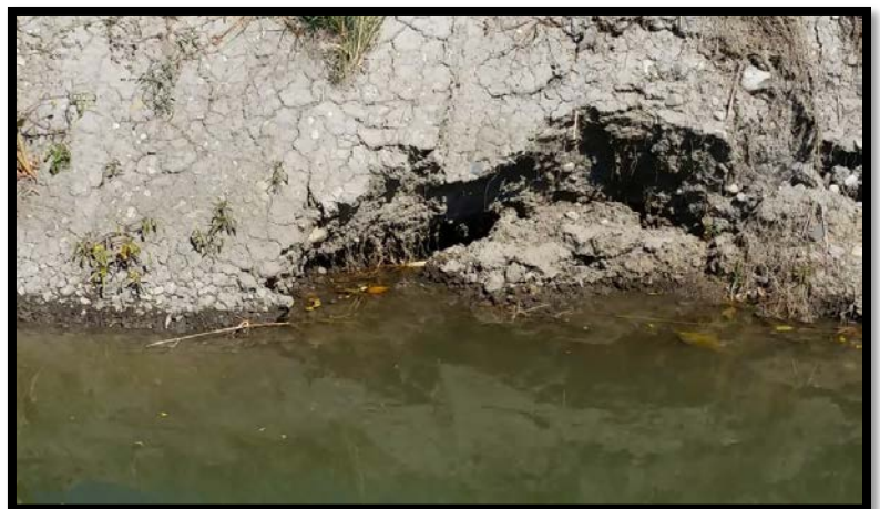
Photo 2 Hammond East Canal Bank Eroding
