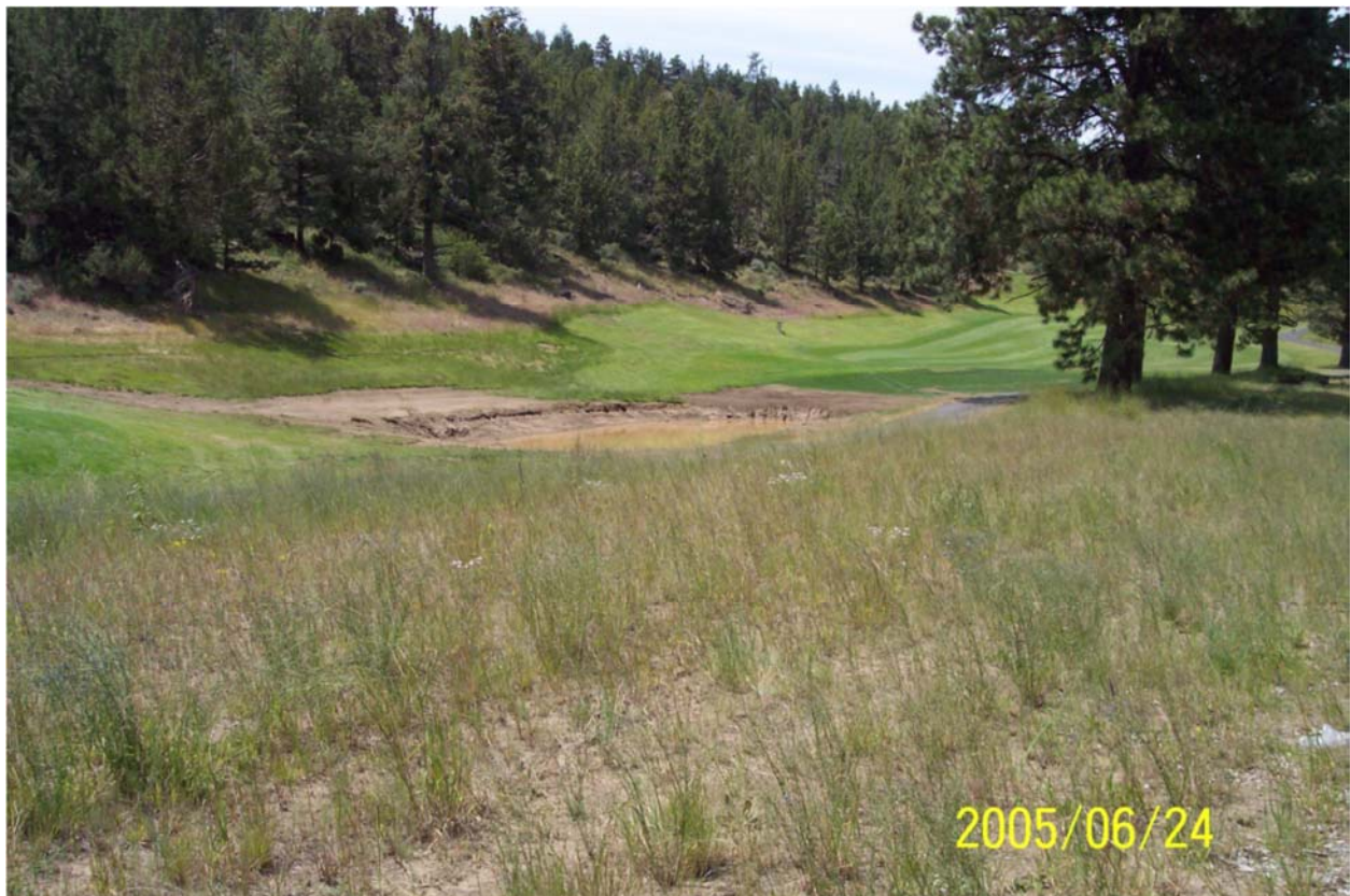
Figure 3: Typical Post-Construction View of Buried Pipe Alignment (photo from Bend Feed Canal Piping Project)
