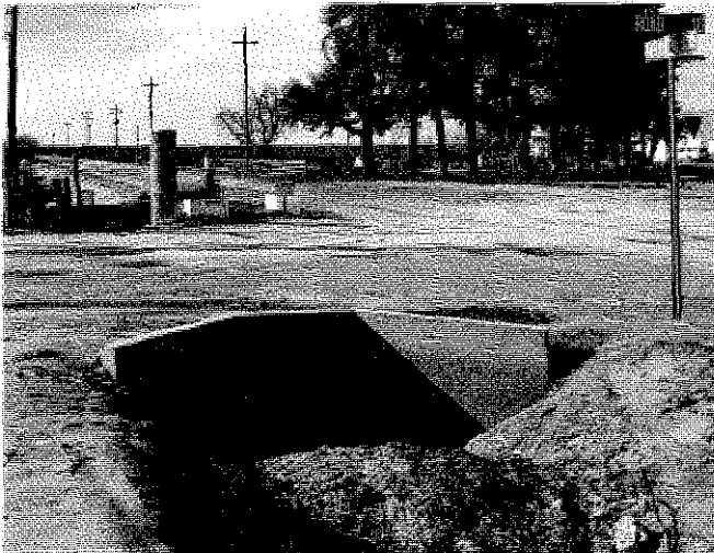
Existing culvert crossing Avenue 15 filled with sediment from unstable, sandy canal soils.
