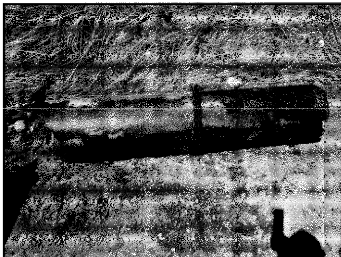
PHOTO 3 55-YEAR-OLD ASBESTOS CEMENT PIPE
