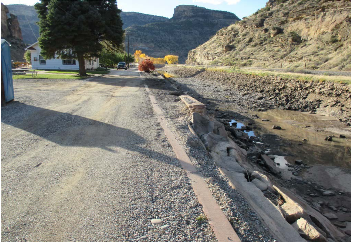
Figure 4. General setting and existing condition of the top 500 feet of the Canyon Canal; looking down canal.
