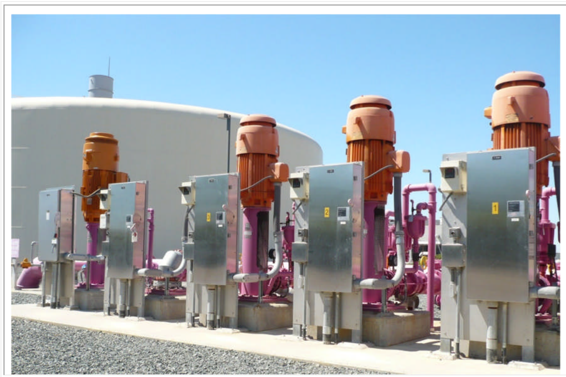
RWF Recycled Water Pump Station – 200 HP Distribution Pumps
