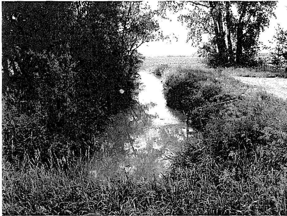
Photo 11 - High Canal 1st Y at the beginning of turn out heading north on west side of Co Rd. 350. High vegetation area and tree growth.
