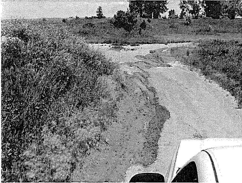
Photo 3 - High Canal just before the siphon showing severe seepage surfacing from the canal banks.
