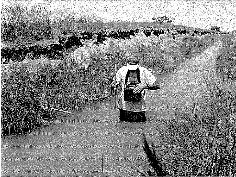
Photo 1 - Beginning of High Canal to Co. Rd. 350. Water flow measurements being done. Erosion of soils on the left side of the canal.
