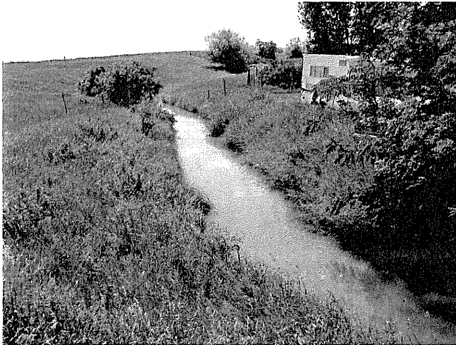
Photo 6 - High Canal just before the last bend to the Co. Rd. 350. Severe vegetation growth on both sides with very slow water flow.
