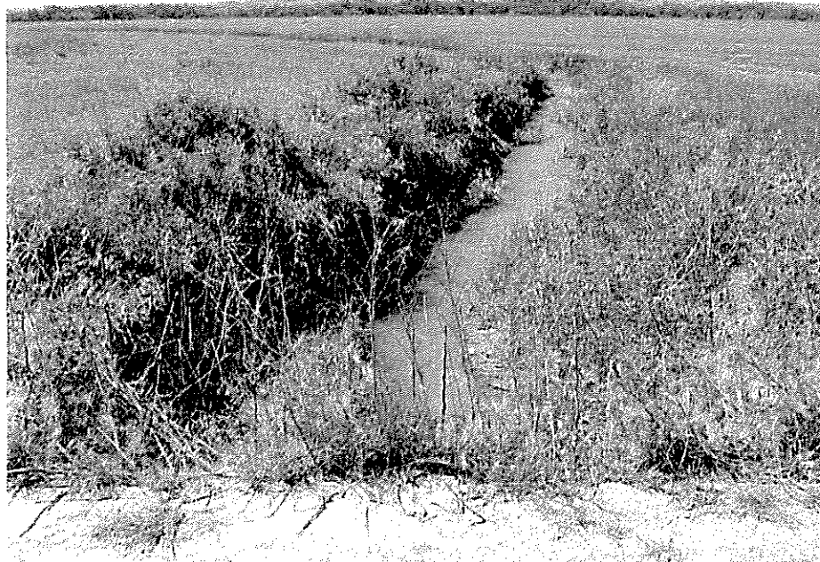
Photo 8 - High Canal heading west at swift current showing ditch bank erosion and infested with weeds.
