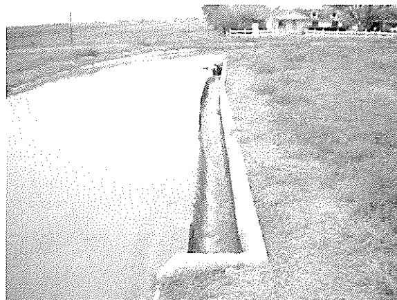
40' Long Overflow Structure
