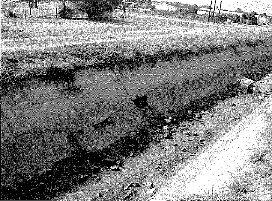
Picture 1. Visible horizontal cracks just North of FM 495.
