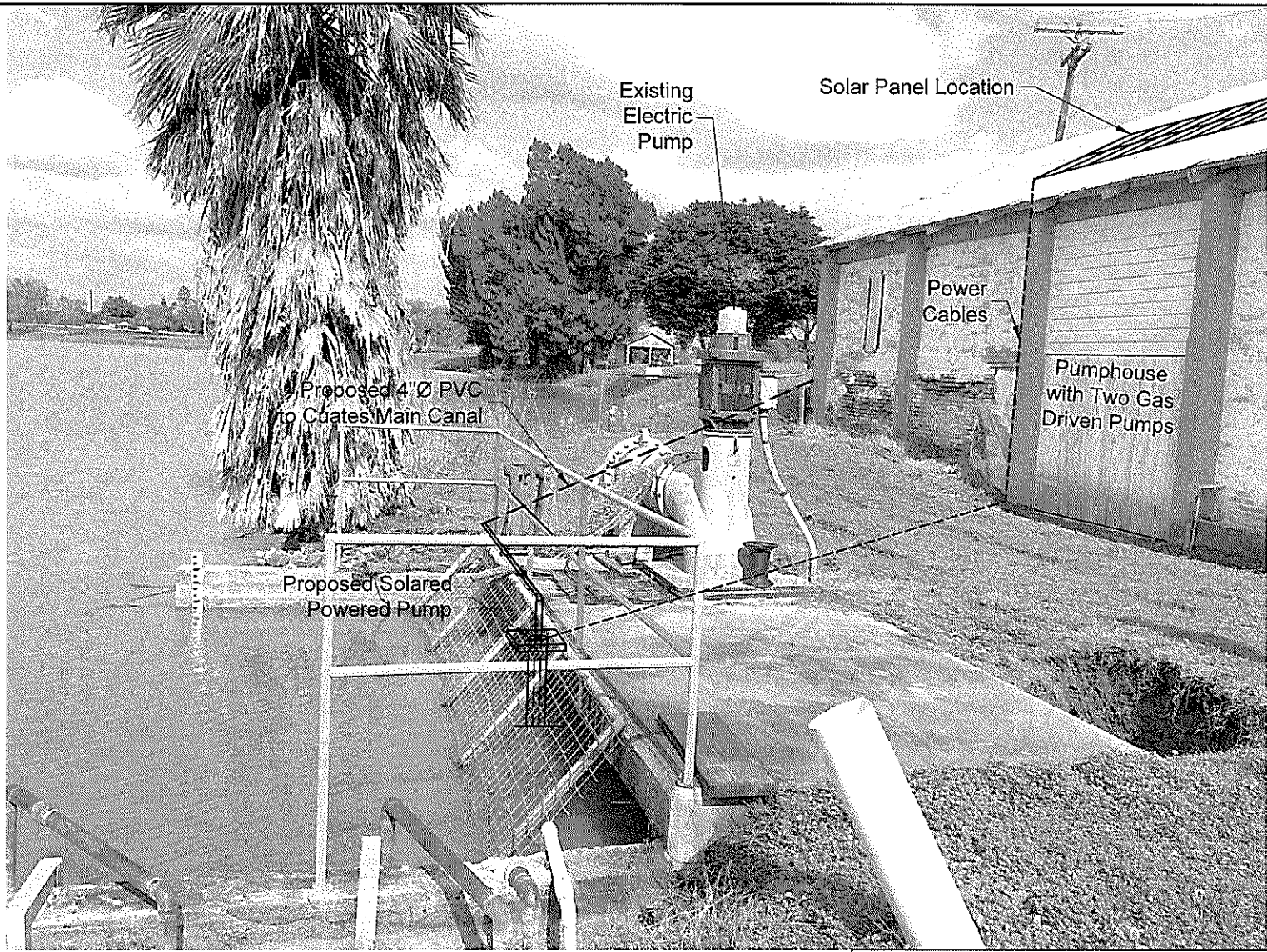
Cameron County Irrigation District No. 6 WaterSMART Grant Application FY2015 Figure 4.4 Photograph of Solar Powered Pump Location Job No.: 408-004 Date: 01/07/2015
