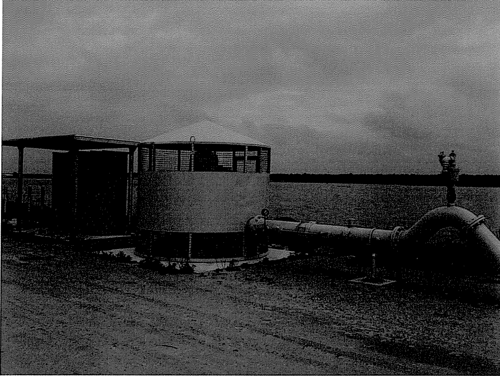
Typical RRBWSD Well 300 HP – 3000 gpm @ 300' TDH Total Depth 475'
