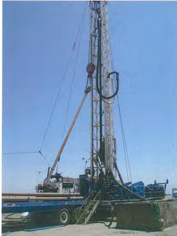
Figure 9: Stockdale West Well Construction Will Be Similar to the Strand Ranch Wells (shown here)
