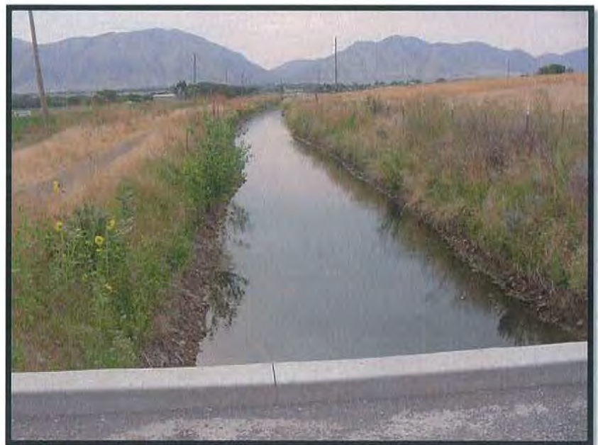
Canal with 80 year old liner
