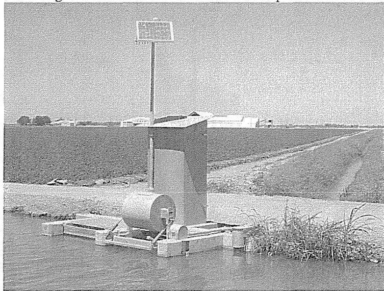
Figure 20. Automatic Spillway using an ITRC Flap gate connected to SCADA to monitor spill flow.
