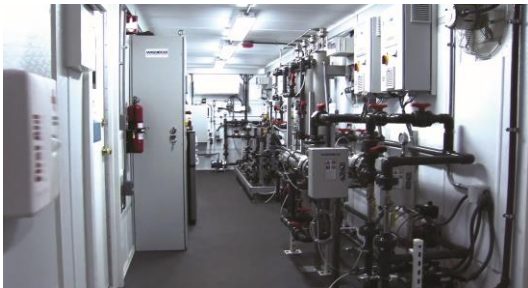
Figure 4 WE&RF Project 15-10 Oxelia Pilot Unit from Xylem.
