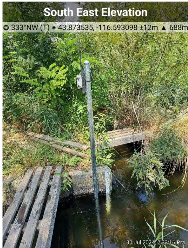
Photo 2 – Example of RTM technology installed by District personnel.
