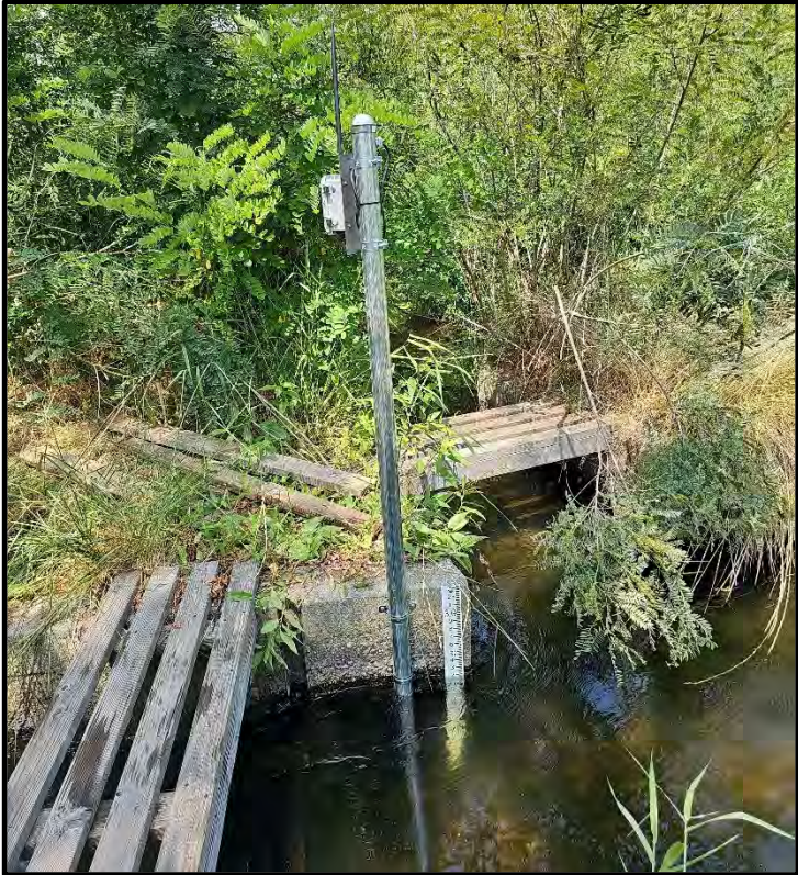
Photo 1 RTM Installed by District Staff
