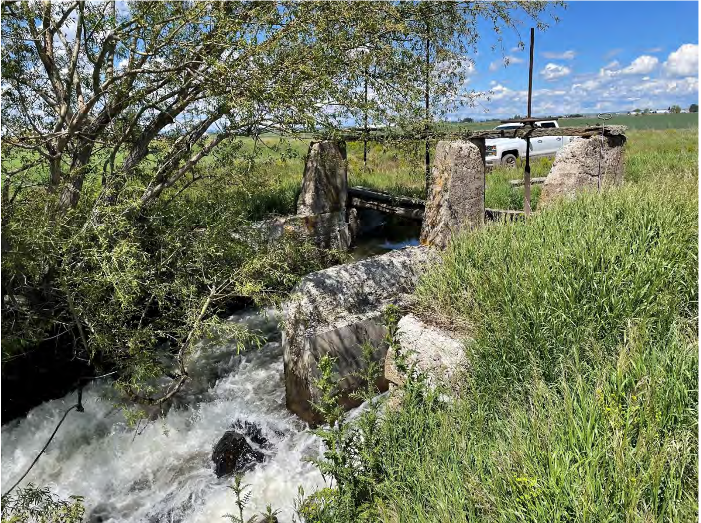
Woodmansee Johnson Canal Diversion Dam-Water Control Structure to be Replaced and Automated
