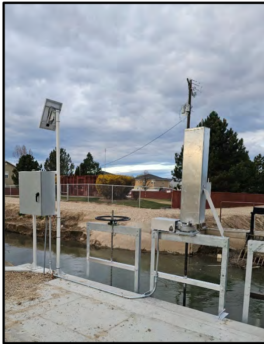
Photo 1 – District Installed Automation Site
