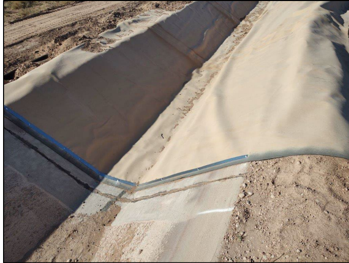
Figure 4. Photo of liner attached to existing concrete in the vicinity of Lateral 26.5.
