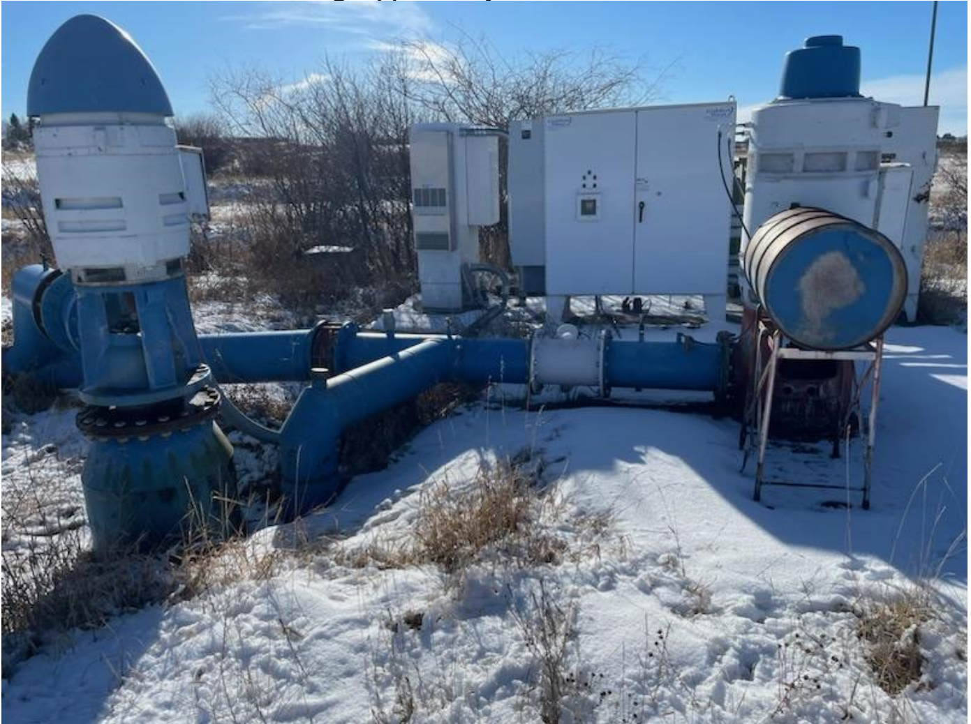
Pumping Station with Flow Meter
