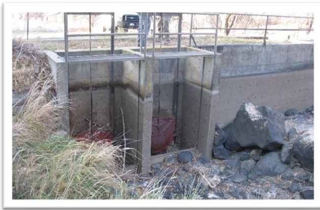
Left: Waldvogel Canal headgate on pond side.
