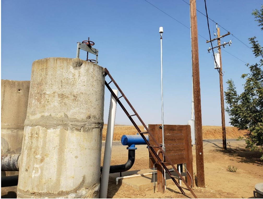
Figure 5: Typical RTU Installation
