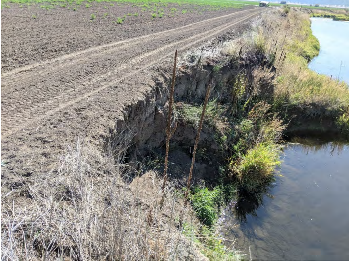
Bank erosion along the Crooked River on King Ranch; bank wasting can add significant amounts of soil and sediment to the river at unnatural levels.
