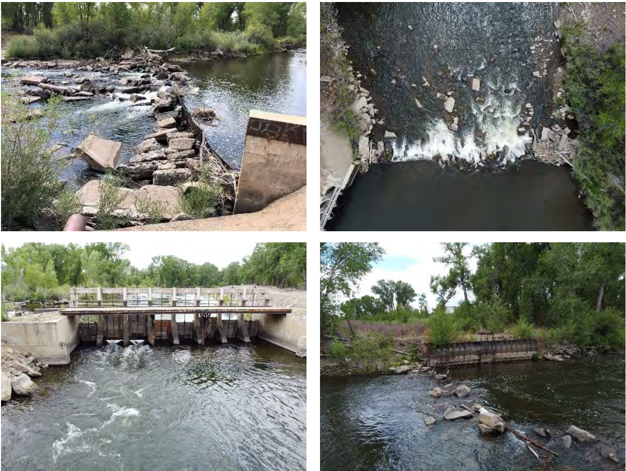
Figure 6. FUC diversion (upper left); aerial view of FUC diversion (upper right); FUC headgate infrastructure looking upstream (lower left); Rio Grande #1 Ditch diversion and headgate (lower right).
