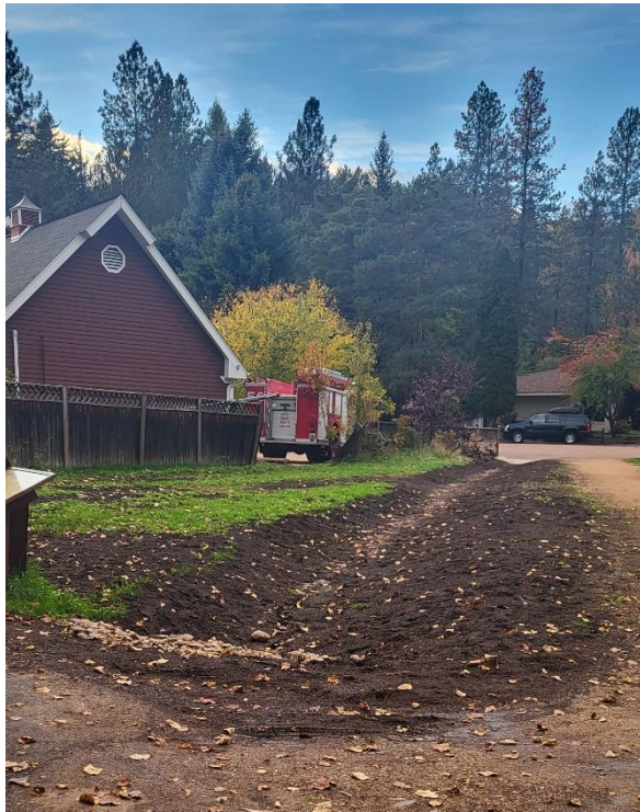
Figure 5 Recently constructed bioretention swale in the lower Rattlesnake neighborhood. Photo credit: Matt Trentman 2023
