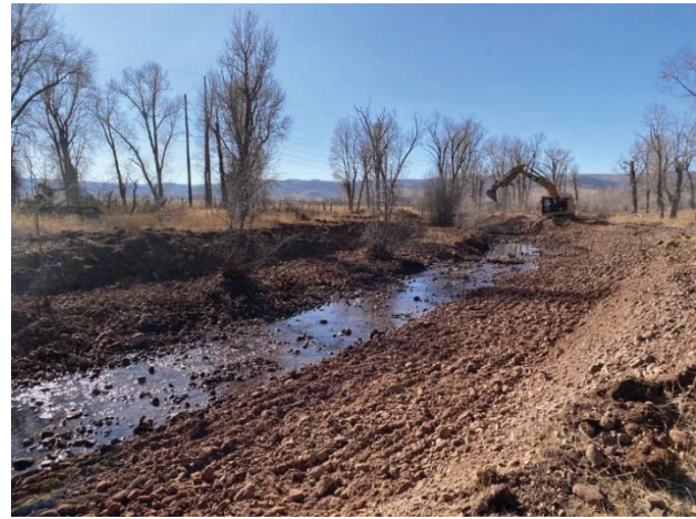
Figure 7: Stream restoration techniques that increase floodplain connectivity, stream and bank stability, and riparian vegetation such as those being used on the Lower Swift Creek Restoration and Stabilization Project result in multiple watershed benefits.
