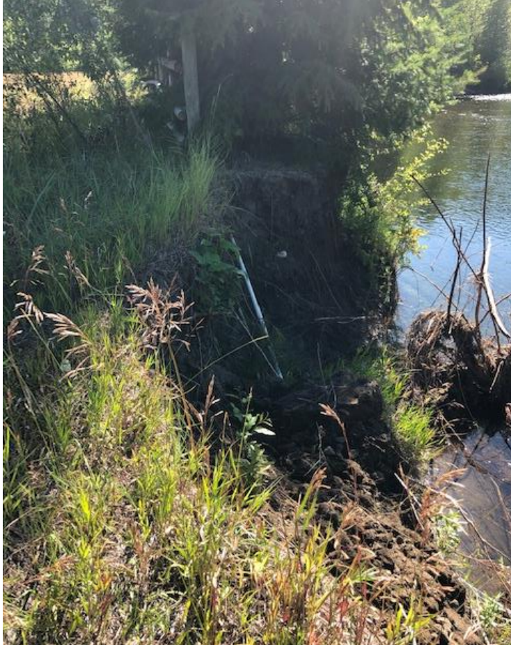
Figure 3. Photo of active bank erosion on Fromm property
