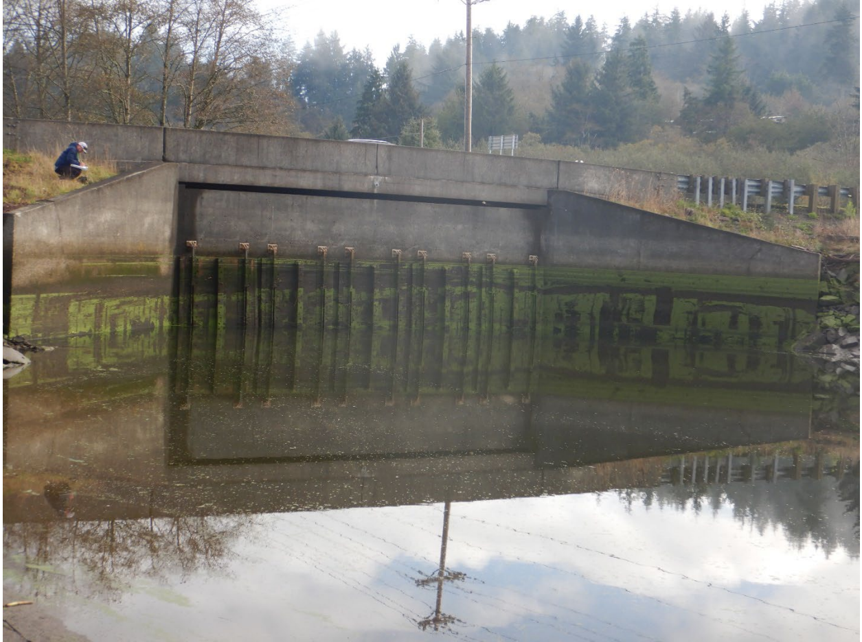
Figure 5. Gallagher Slough tide gates (5) to be replaced with a muted tidal regulator gate.
