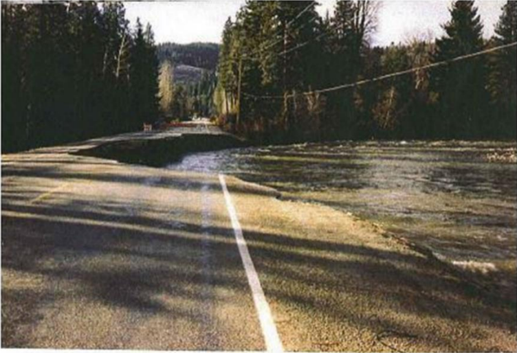
Figure 3, Roadway erosion in 1995.
