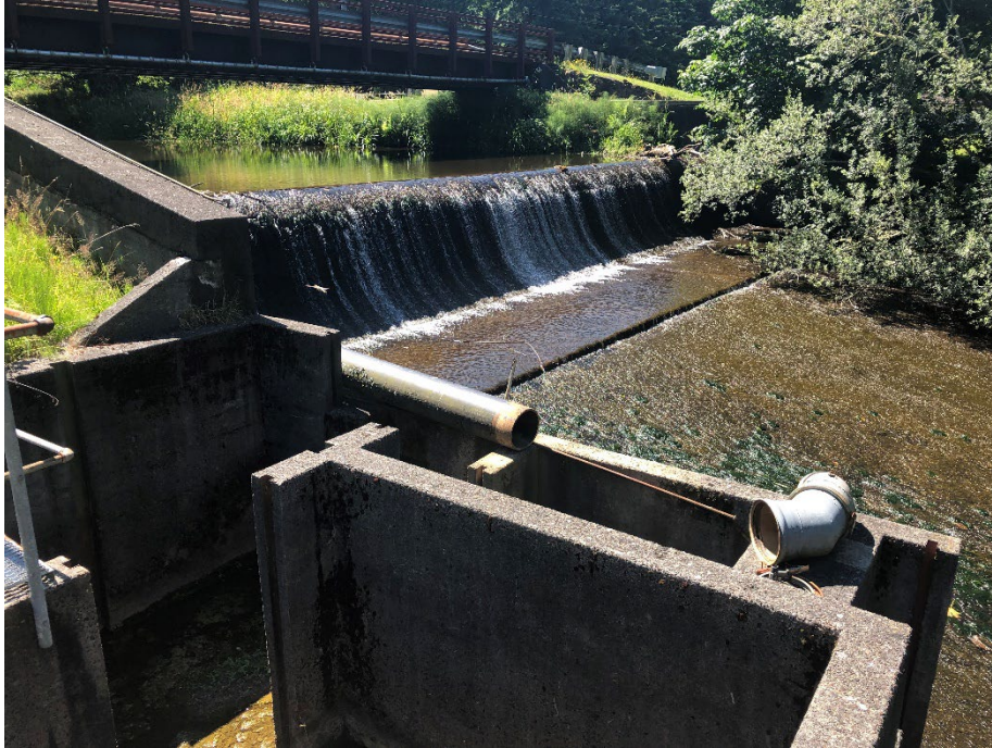
Figure 3. Cross sectional view of the Ogee Crest dam and appended concrete apron located on North Fork Klaskanine River, Oregon.
