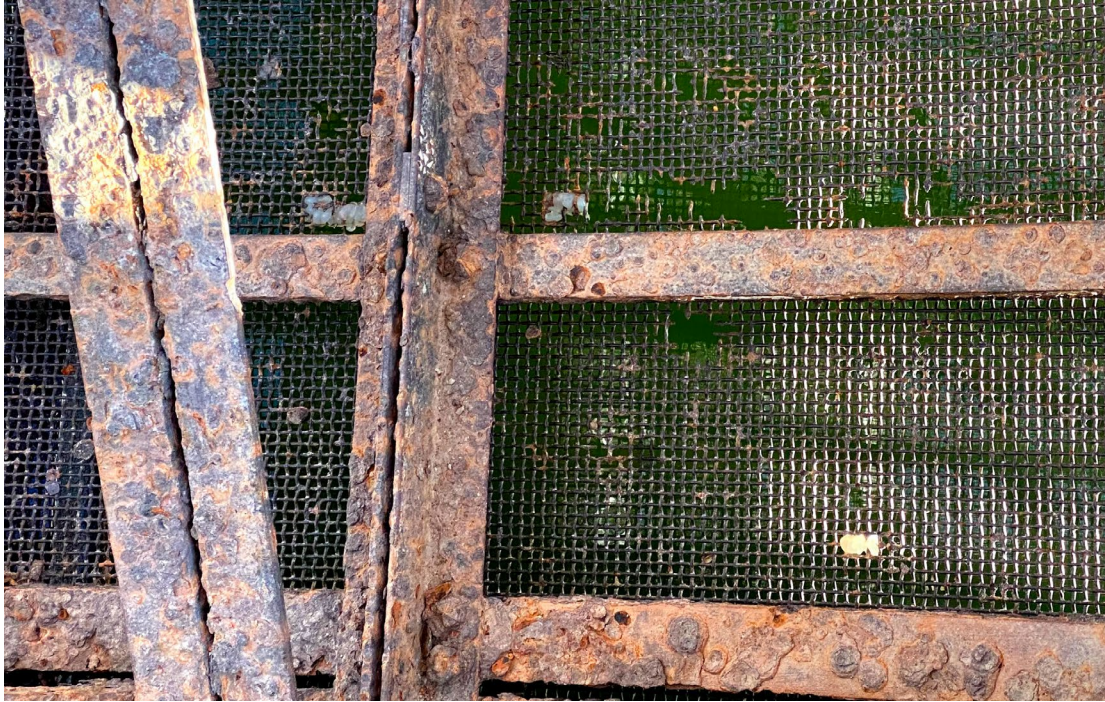
Screen Material with Extensive Damage resulting in Open Spaces >1/4."
