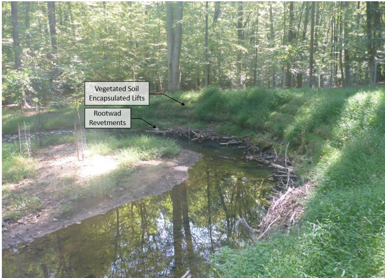
Figure 3: Example of Rootwad Revetments with SELs in Rockville, Maryland
